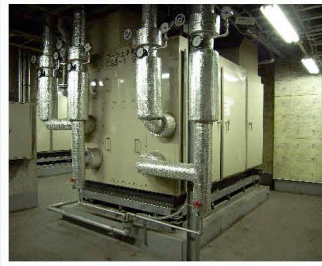
Cogeneration at Super-high Rise Building C
